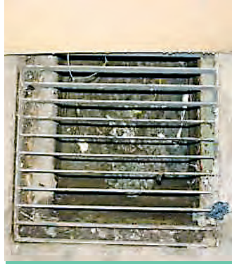
Drains and sewage systems must be built with proper traps and ventilation.
